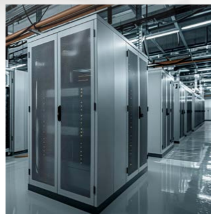
Data centers require reliable, rapid-response power to protect infrastructure and prevent disruptions that could compromise data.
